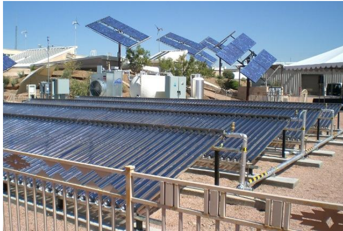
Salt River Project testing solar air conditioning with Guard.
