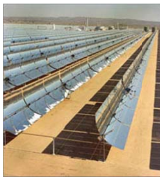
Figure 2: Parabolic trough system.
