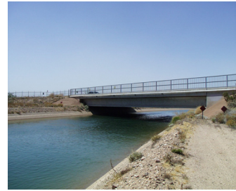
Figure 4: View NW from the north side of the canal, looking at the Via Linda bridge (here, Via Linda runs E/W). This is the area of greatest subsidence of the canal (1.5 feet in past 10 years). There is ~2.5ft of freeboard at this location. Photograph by J Ramón Arrowsmith.
