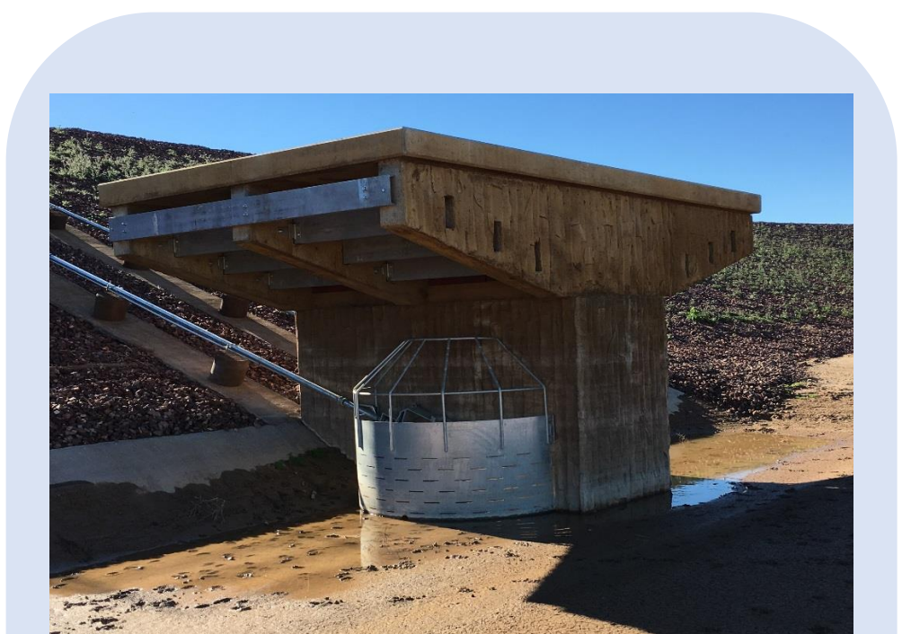
Fig 6: Principal Outlet Structure at White Tanks 4. Stormwater is discharged via slide gates and high stage inlets
