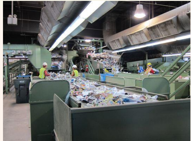
Figure 1. Phoenix recovery facility (Photo: City of Phoenix Department of Public Works)
